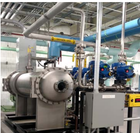
New Ozone System installed in 2017 at CLCJAWA
